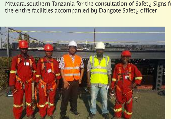
Sign Industries CEO with installation team for the project of Kilimanjaro International Airport during the installation of LED signs under BAM International.
